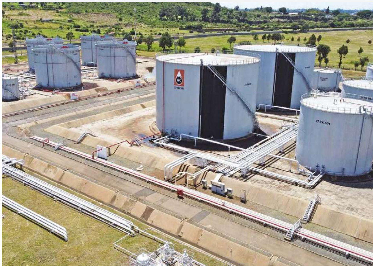
Kenya Pipeline Company's Eldoret pump station on October 18, 2023.
