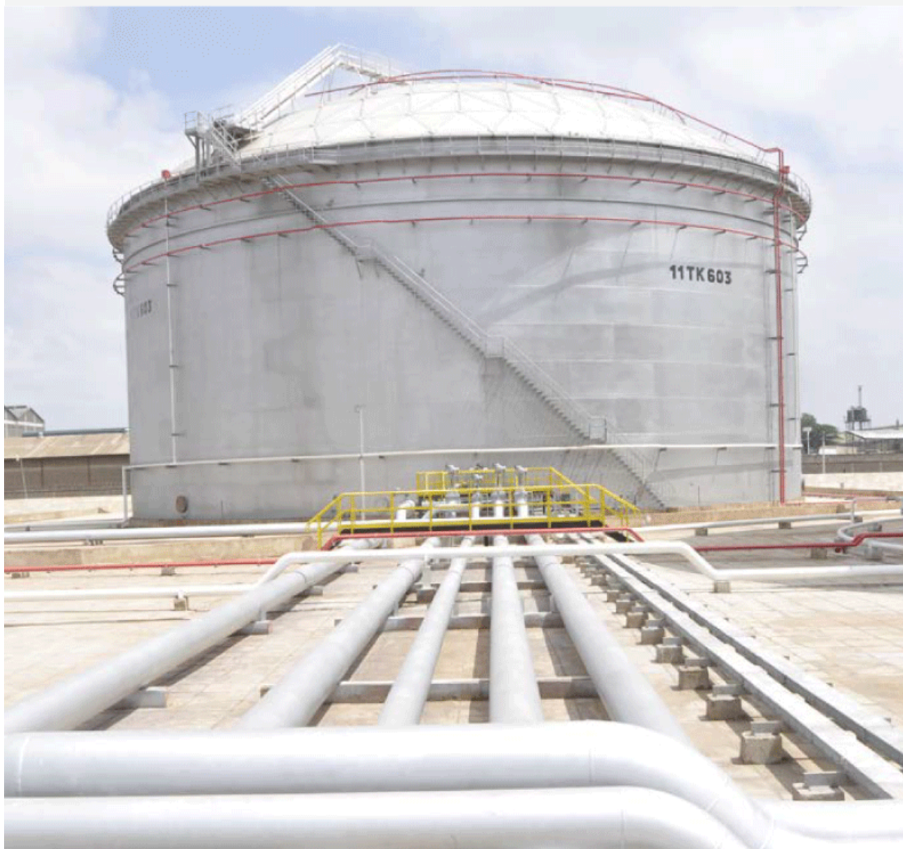
Storage tank at Nairobi Terminal
