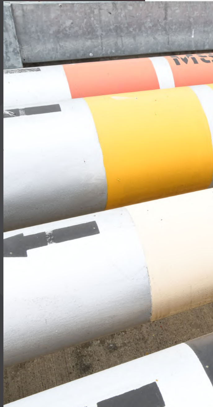
Inter-sites pipelines at Kisumu (PS28) Depot
